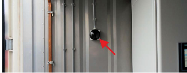
Process Stop Button in ESI Room
